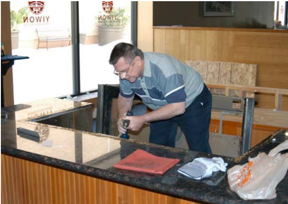
Gene Spann undoing the support frames as we work to disassemble and take out of the restaurant.
