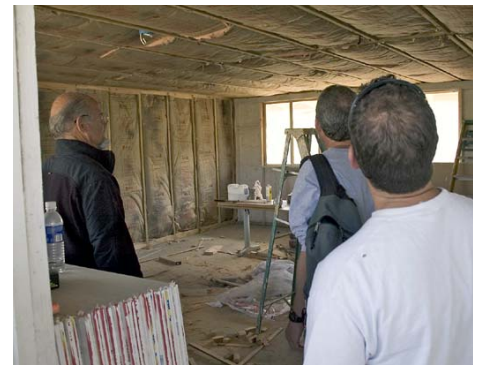
Arriving at the school and the bare, but insulated classroom ready for drywall.
