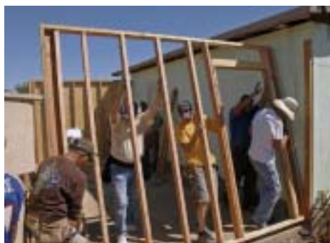
The framing goes up on the concrete pad Norm had laid previous to this trip.
